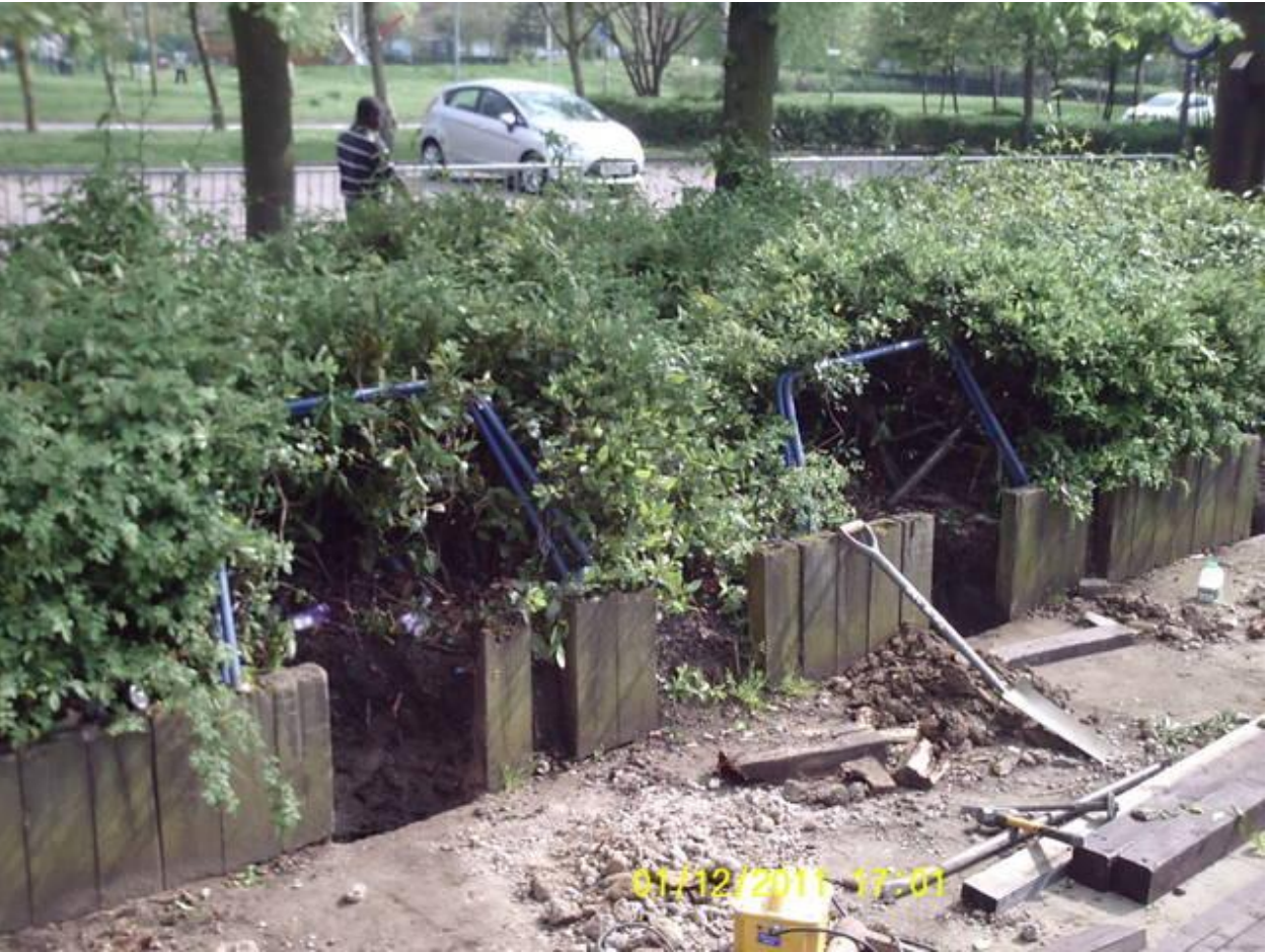
Initial demolition of the fenced off area between the Fishermead Trinity Centre and the Co-Operative Store.
